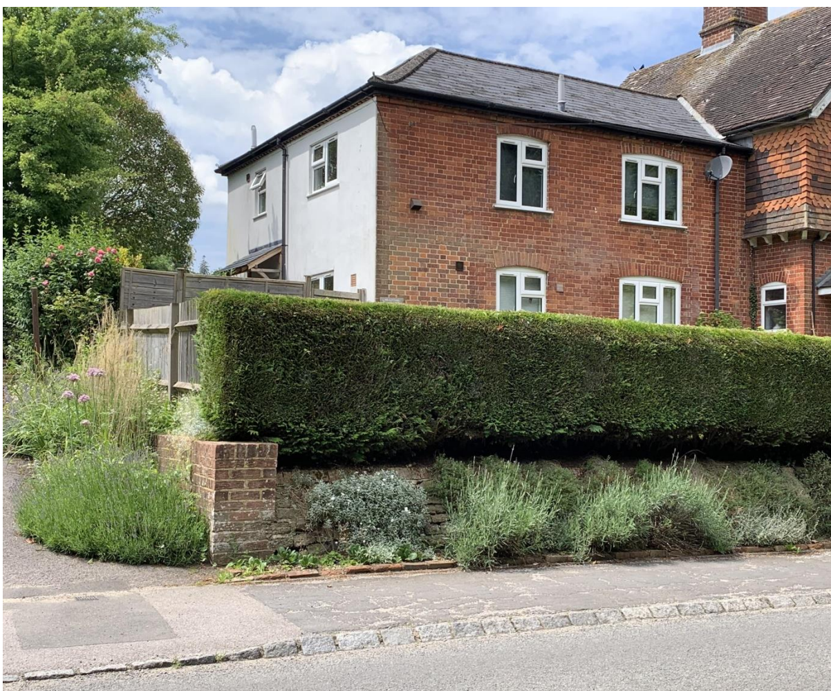
Figure 2: Brickwork wall, brick pier over 850mm high and the traditional Bargate stone retaining wall.
